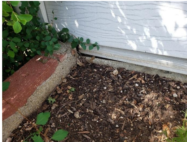
Dirt in the planter box is adjacent to the house wall. A layer of sheet metal is seen possibly protecting the house from moisture.
