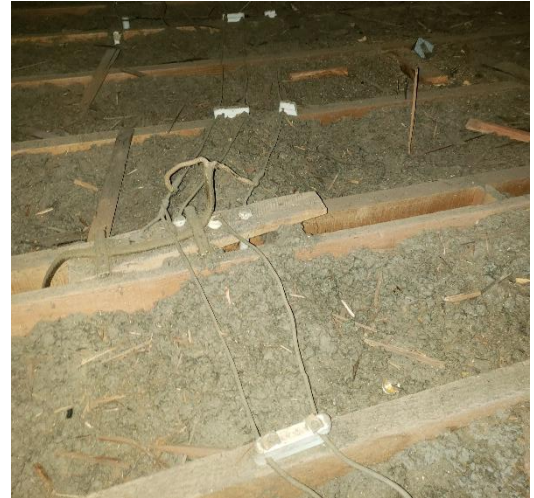
Cloth-sheathed wiring in the attic.
