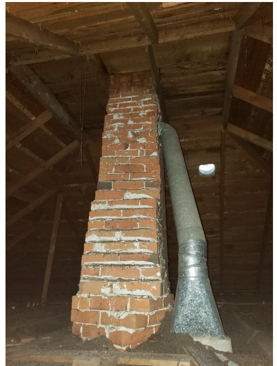
The water heater vent enters the chimney in the attic.
