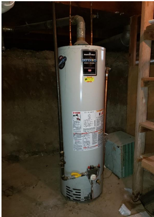
40-gallon gas-fired water heater in the basement.
