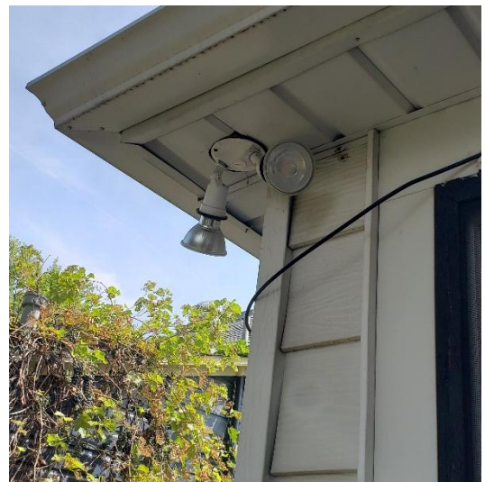
Flood light in the northwest house corner.
