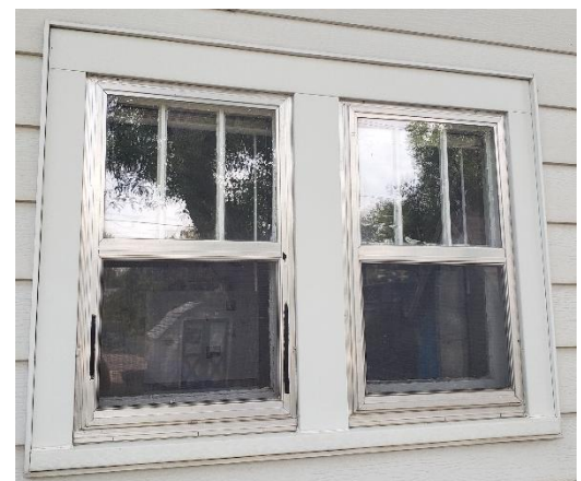
Metal wrapped window trim & typical j-trim.
