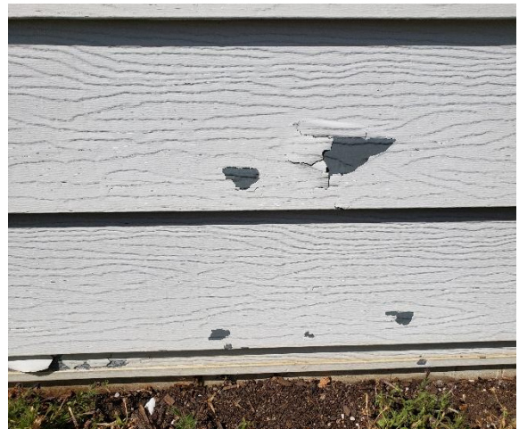
Chipped paint finish common for metal siding.
