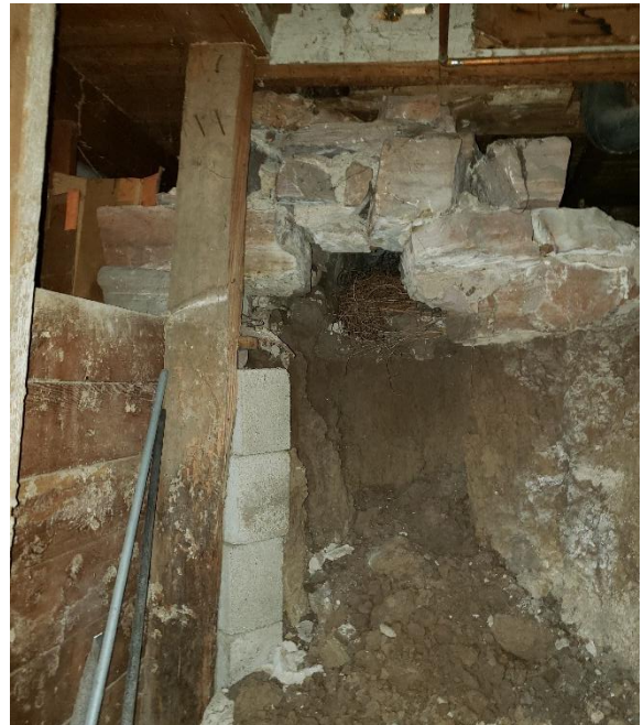
Original stone foundation undercut by sluffing soil.
