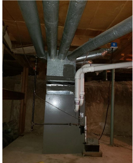
Gas furnace that sits on the concrete basement floor.
