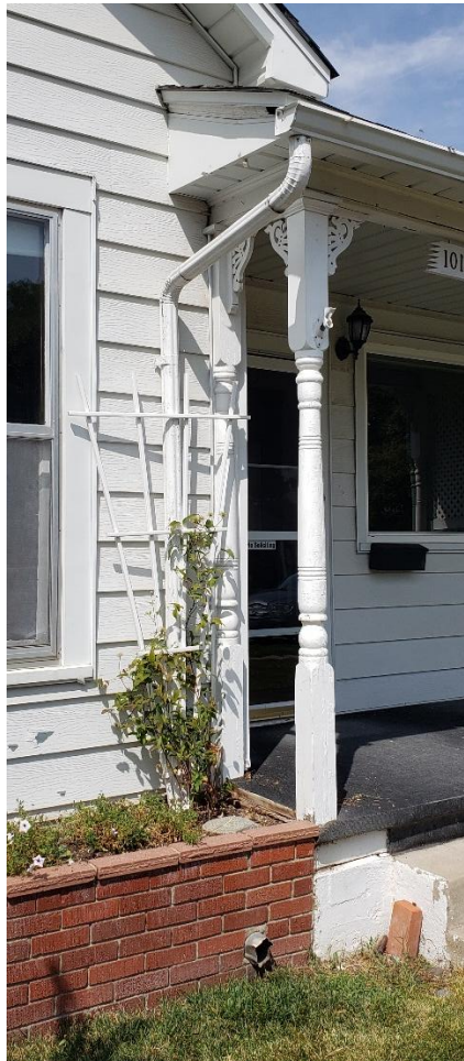
Round downspout buried in brick planter.
