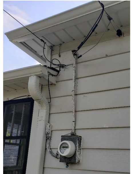
Electrical meter on the west side of the house.
