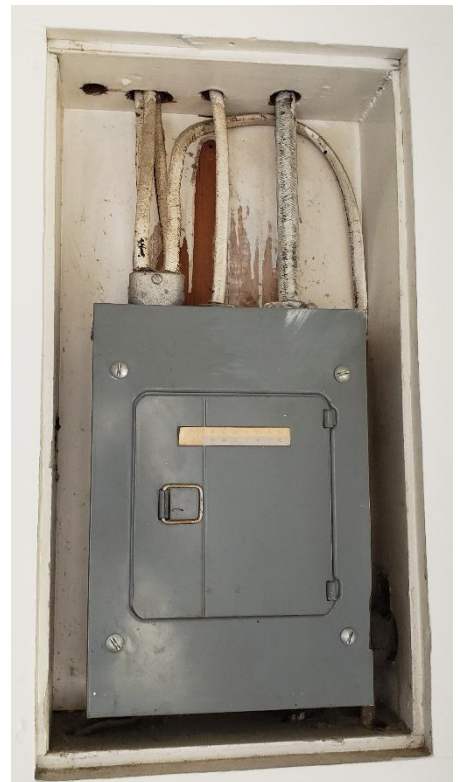
Electrical panel in the mudroom.
