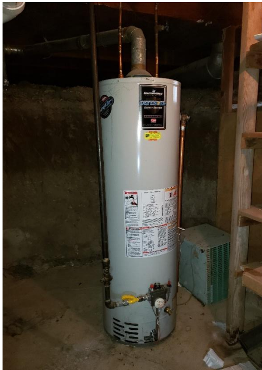
40-gallon gas-fired water heater in the basement.
