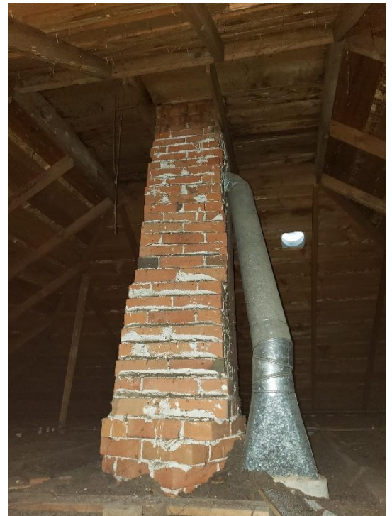
The water heater vent enters the chimney in the attic.
