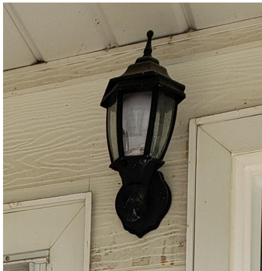
Sconce light at the front door.
