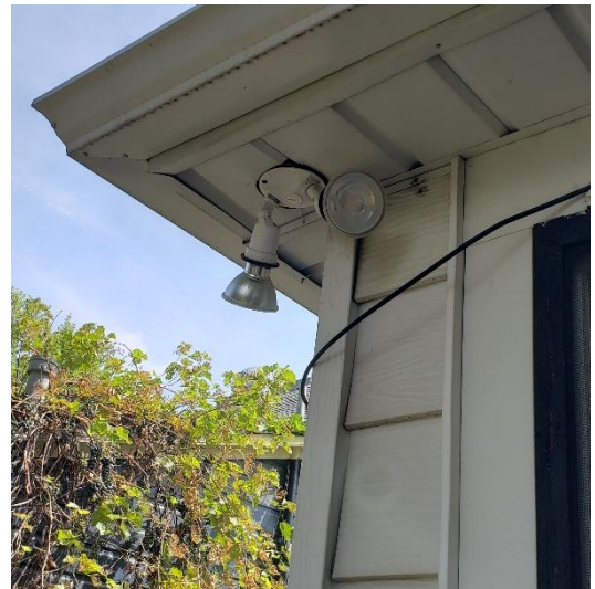
Flood light in the northwest house corner.
