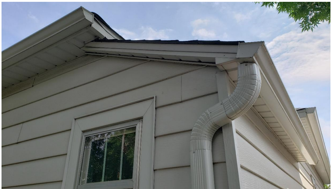
Painted k-style gutters and 2x3 downspouts are located throughout.
