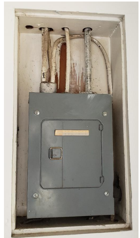
Electrical panel in the mudroom.
