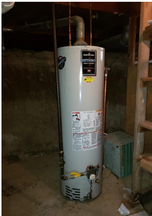
40-gallon gas-fired water heater in the basement.
