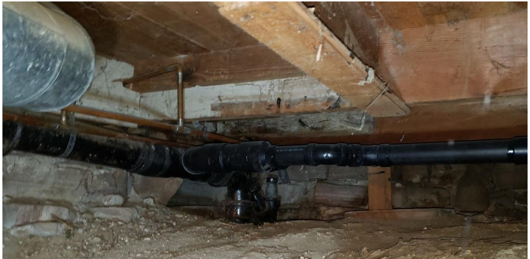
Copper supply lines and abs plastic waste lines to the main cast iron waste line in the basement.
