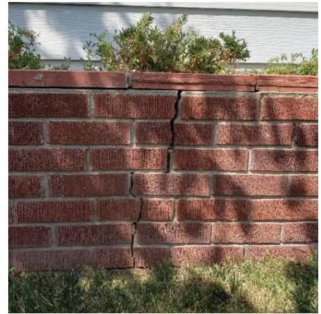
A large crack running the full height of the brick planter box.
