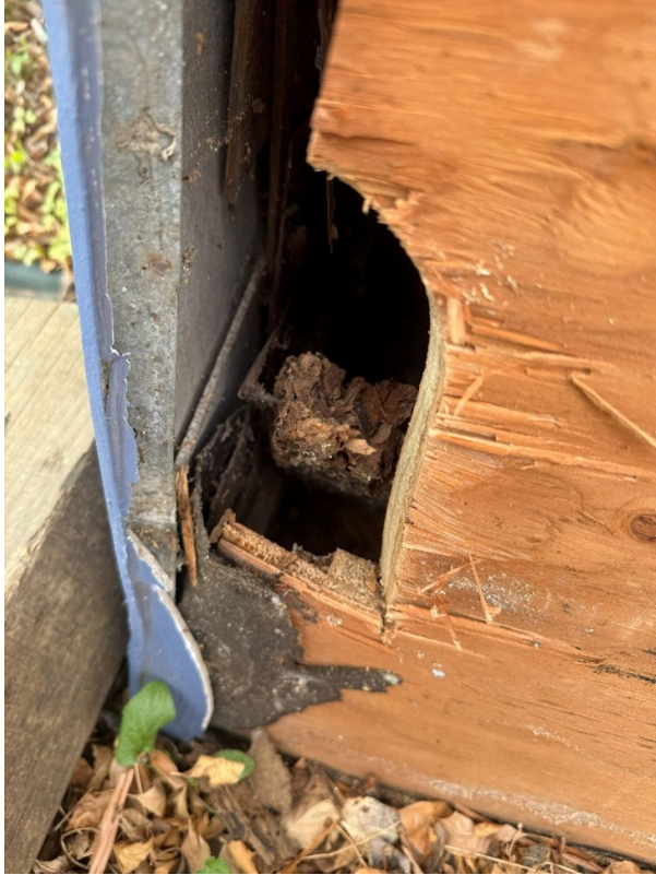
Photo 2 of the exploratory opening, 2026
